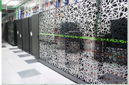
Servers at CNAG
