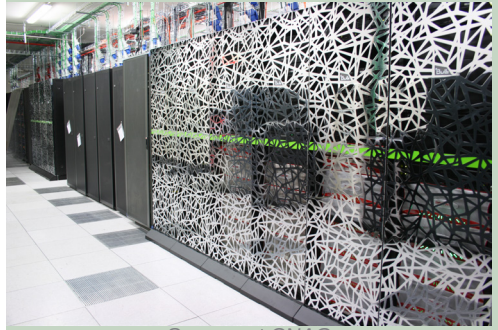
Servers at CNAG
